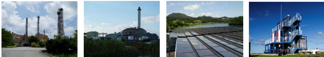
Okinawa Electric Company Kumejima Power Station Diesel Power Generators 7units 16,500kW C-grade heavy oil
